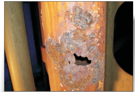
Holes caused by corrosion
